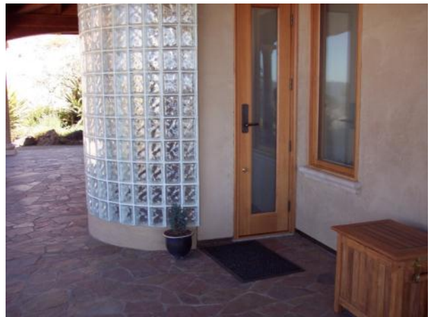
Figure 11 – Glass unit masonry enclosing shower. Note that the sidelite at the right would not require safety glass if the door were hinged on the other side.
