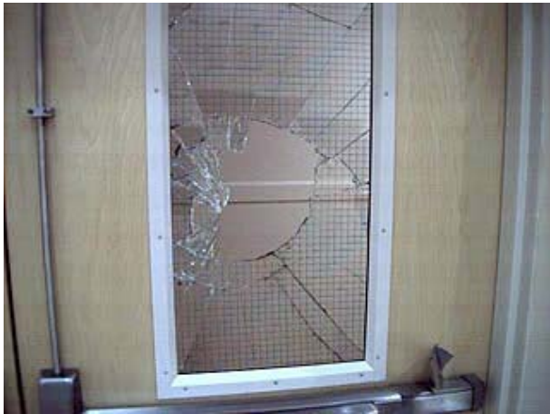
Figure 4 – Vision pane in gymnasium door
