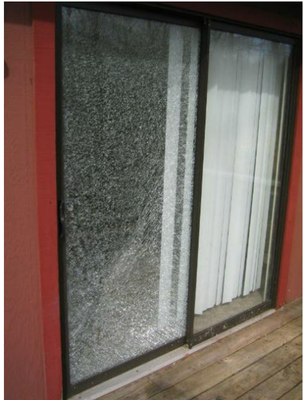
Figure 3 – Broken tempered glass patio door
